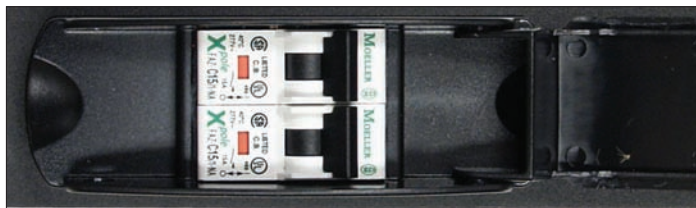
UL 489 hydraulic-magnetic circuit breaker on 30 Amp PDU.
