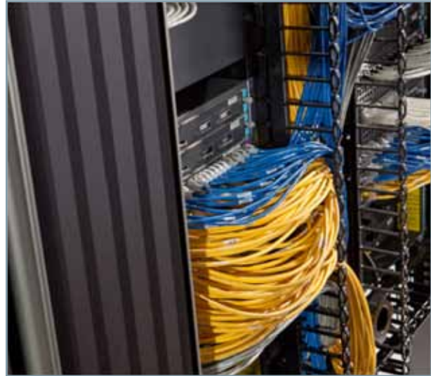
Figure 9. Effective cable management in high-density configuration must prevent stresses on equipment ports while still accommodating MACs
