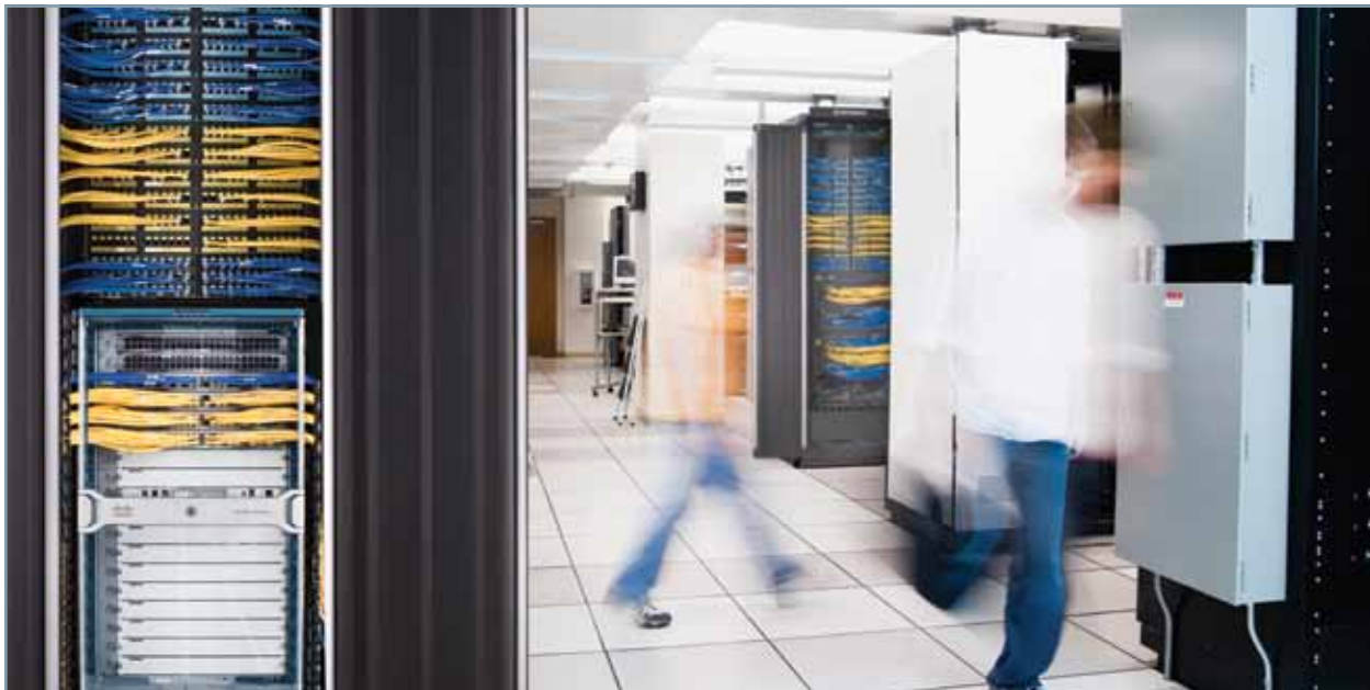
Figure 1. The passive infrastructure – Layer Zero – is a critical layer in achieving a high-performance, reliable network.
